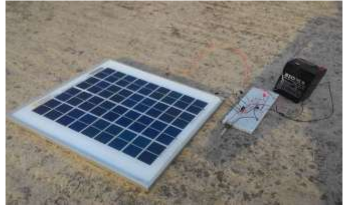
Fig.10. charging of batteries using the solar panel
